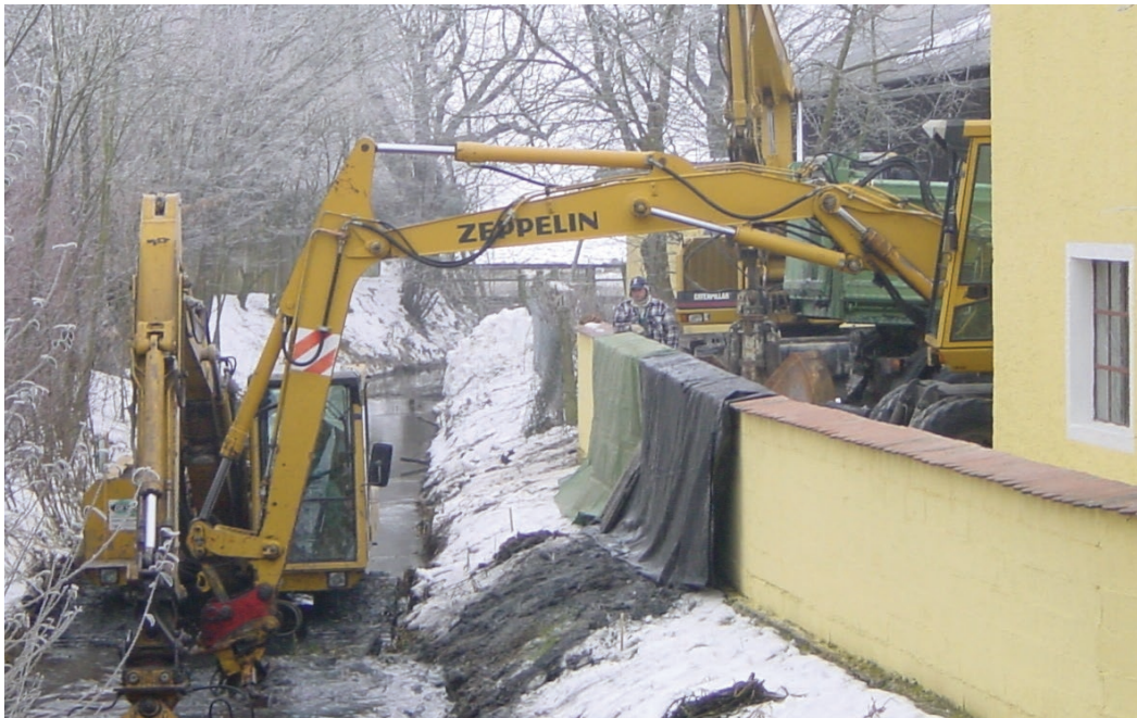
Renaturation of the Great Laaber river in Schierling, Germany. The Mintraching Lohgraben stream runs through the centre of the built-up area and is not freely accessible from any side. The excavator had to drive through a rural estate into the water. Equipped with an extra-wide swamp buggy chassis, the material could be extracted from the middle of the trench and placed to the side by the excavators. With a second excavator, the material was loaded onto one of our trucks.
