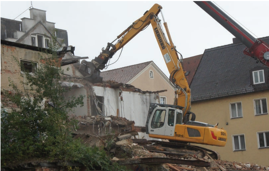
Demolition of the former Red Cross building at Regensburg Stobäusplatz; the project took six months. Centrally located on a Regensburg junction, this project required the utmost caution and sophisticated safety measures so as not to affect traffic or passers-by. The floor area that underwent the work was approximately 30,000 m².
